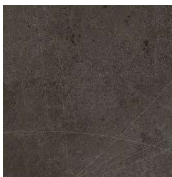
NOT-3995 Scratched Concrete
